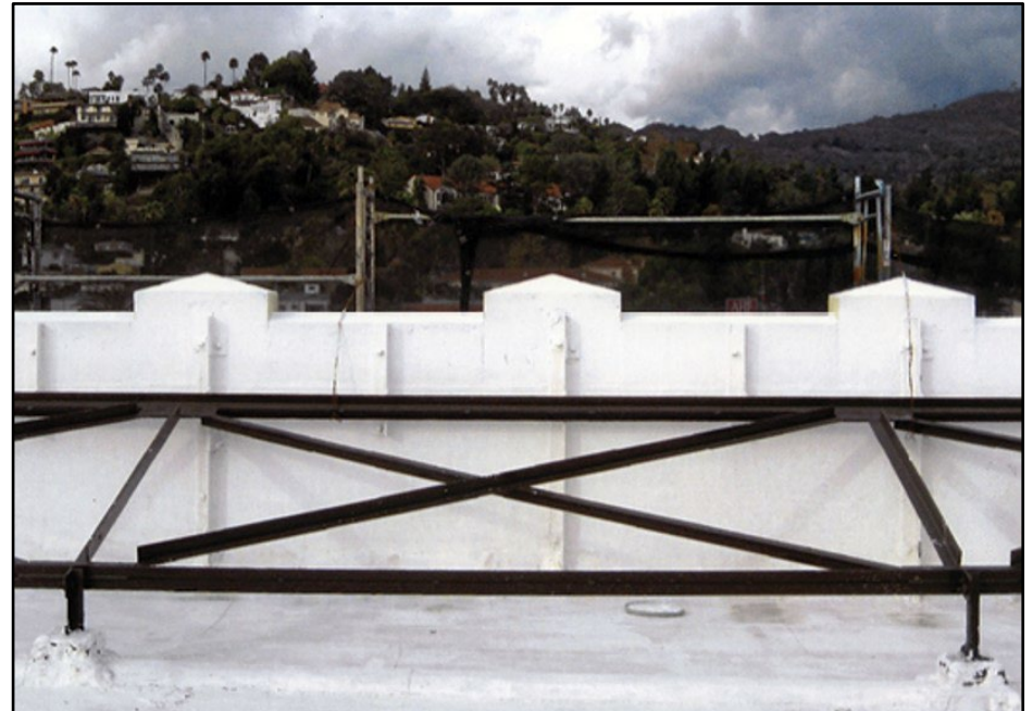
Example of parapet bracing as seen from the roof (Source: National Park Service)
